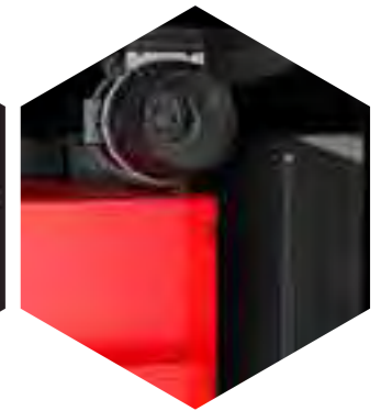
HUMIDITY SENSOR ACTIVATES THE FAN AND HEATER SYSTEMS TO KEEP BATTERIES DRY
